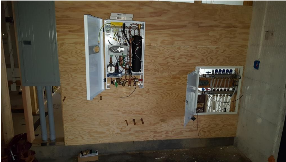
Our Personal NextGen Boiler
